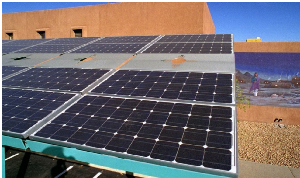
Solar panels at the Pueblo Cultural Center in Albuquerque, NM.
