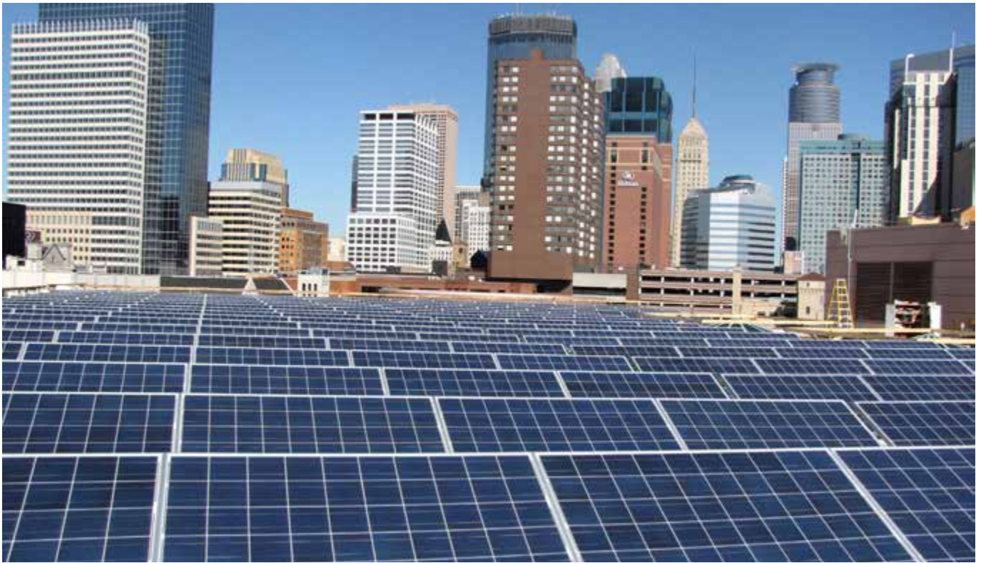
By the end of the first quarter of 2018, America had enough solar capacity – including these panels in Minneapolis, Minnesota – to power more than 10 million homes. 36 Credit: U.S. Department of Energy
