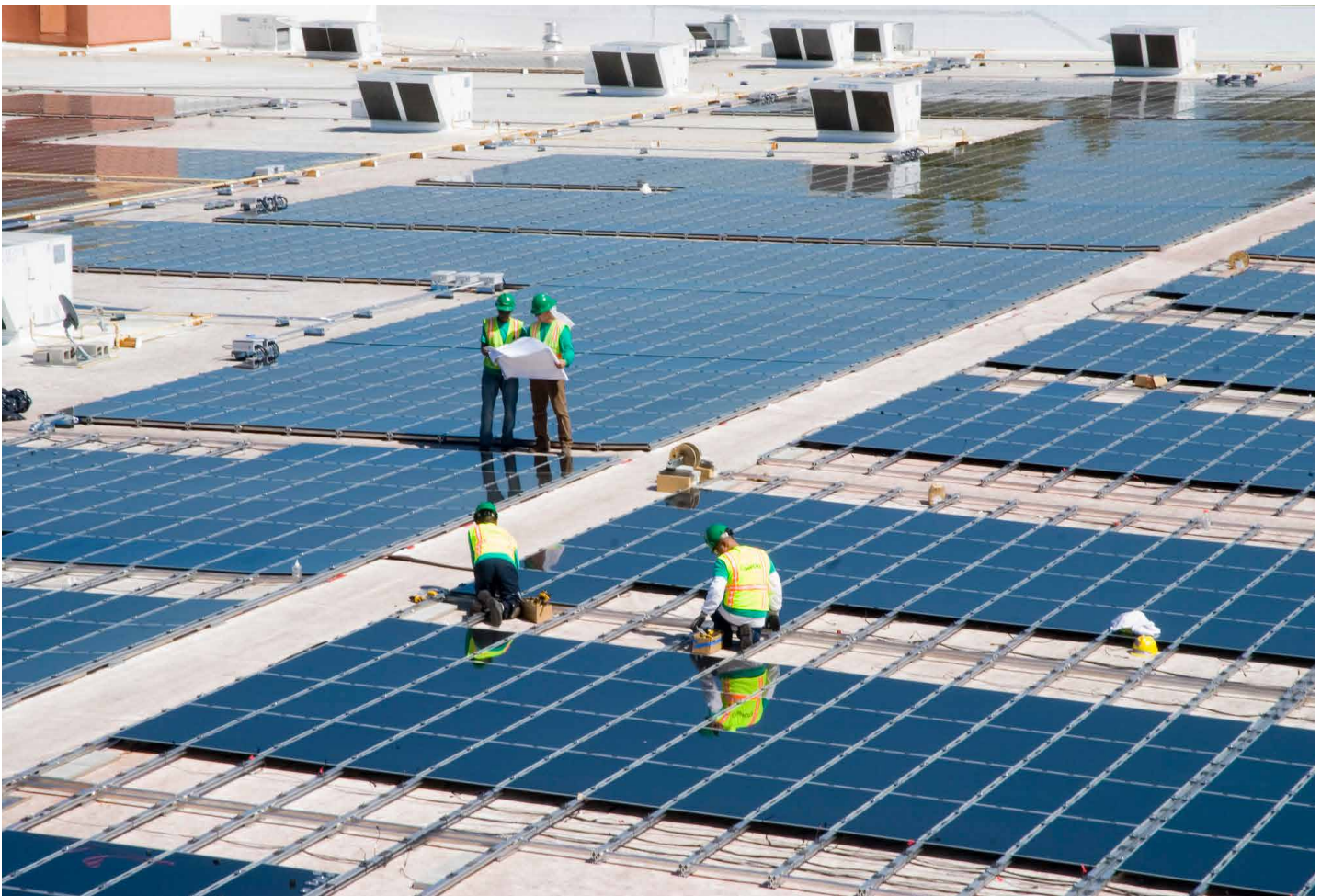
Thin-film solar installation on a Walmart store in Mountain View, California.
