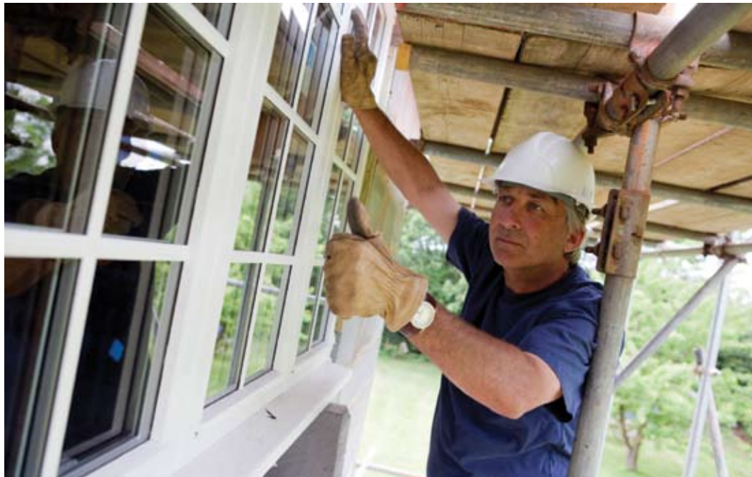
Retrofitting existing homes and businesses for greater energy efficiency is one of the fastest and most cost-effective ways to reduce global warming pollution in the United States. Photo: istock-photo.com, cjp
